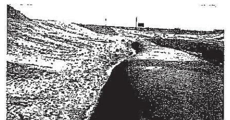
Mirafi® woven geotextile used to construct capping layer over very soft tailings
